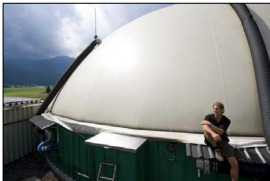
Biogasanlage in Würmlach
